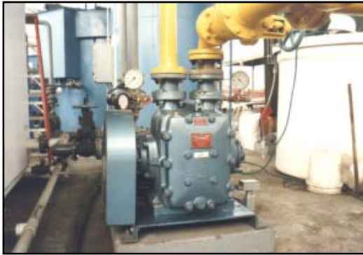
➤ Megator H300 located at a chemical plant
