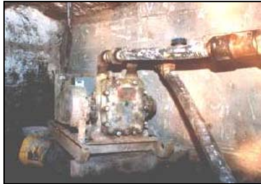
➤ Rugged conditions underground mining duties
