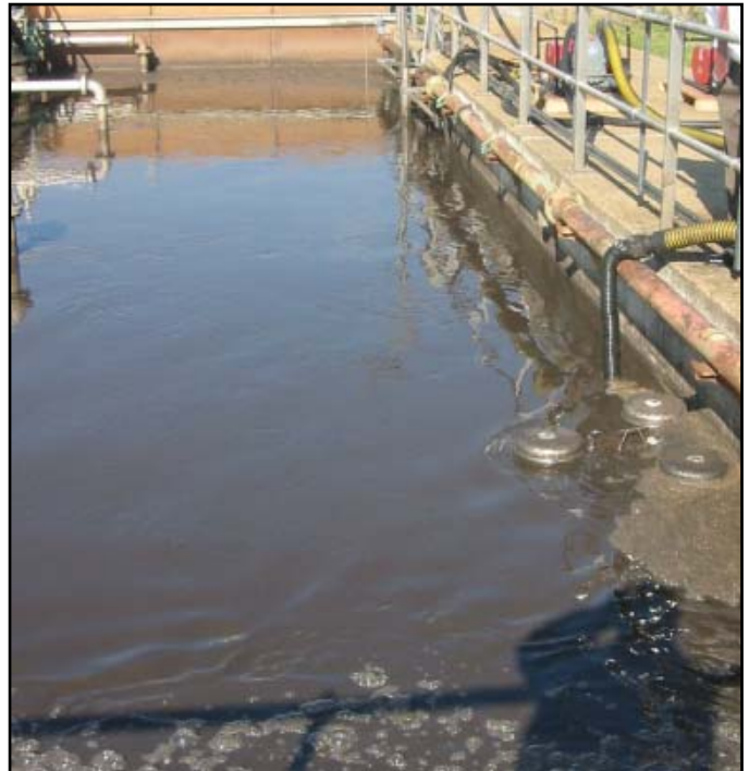
➤ Sewage tank after skimming cycle
